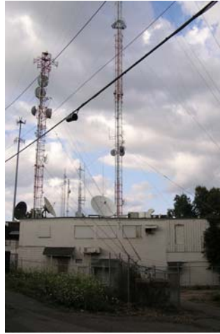
Provin mountain radio site. The building in the foreground is WWLP TV; over 50 years old.
